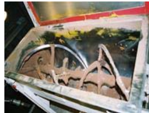
Ribbon mixer before Dry Ice cleaning
